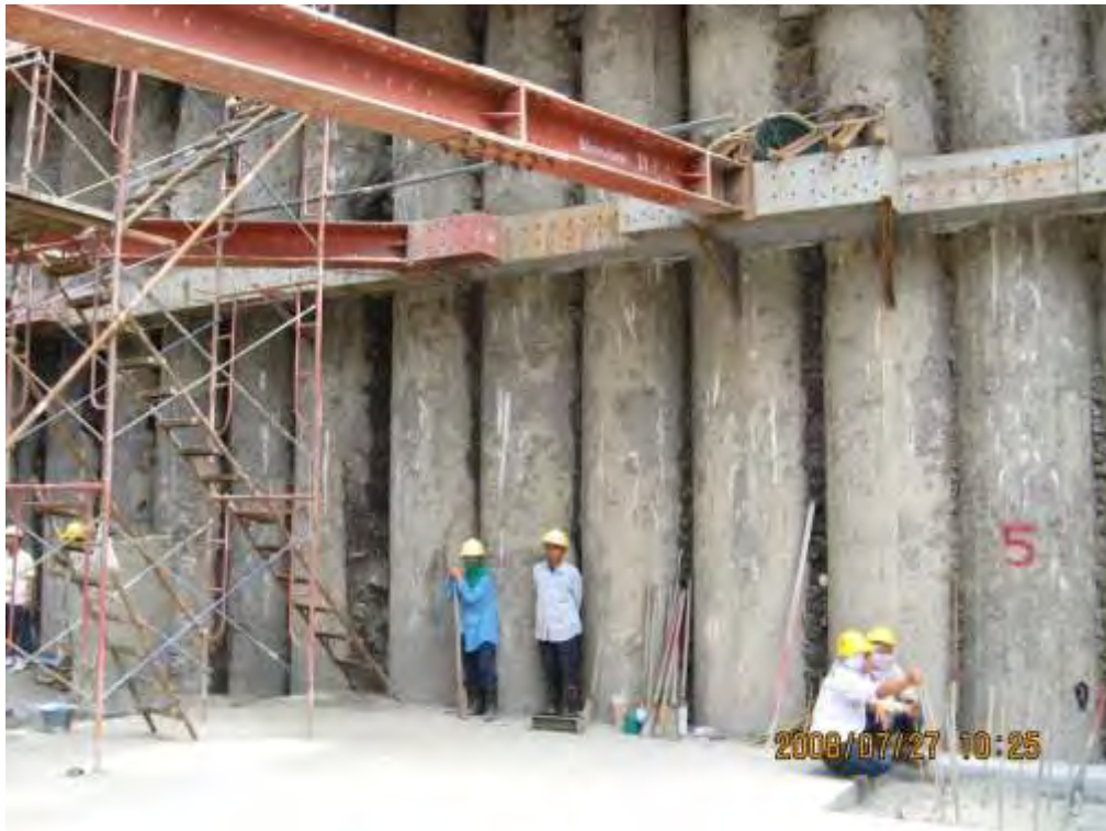
Figure 16 (b). The photographs of the basement construction by means of the contiguous pile wall
