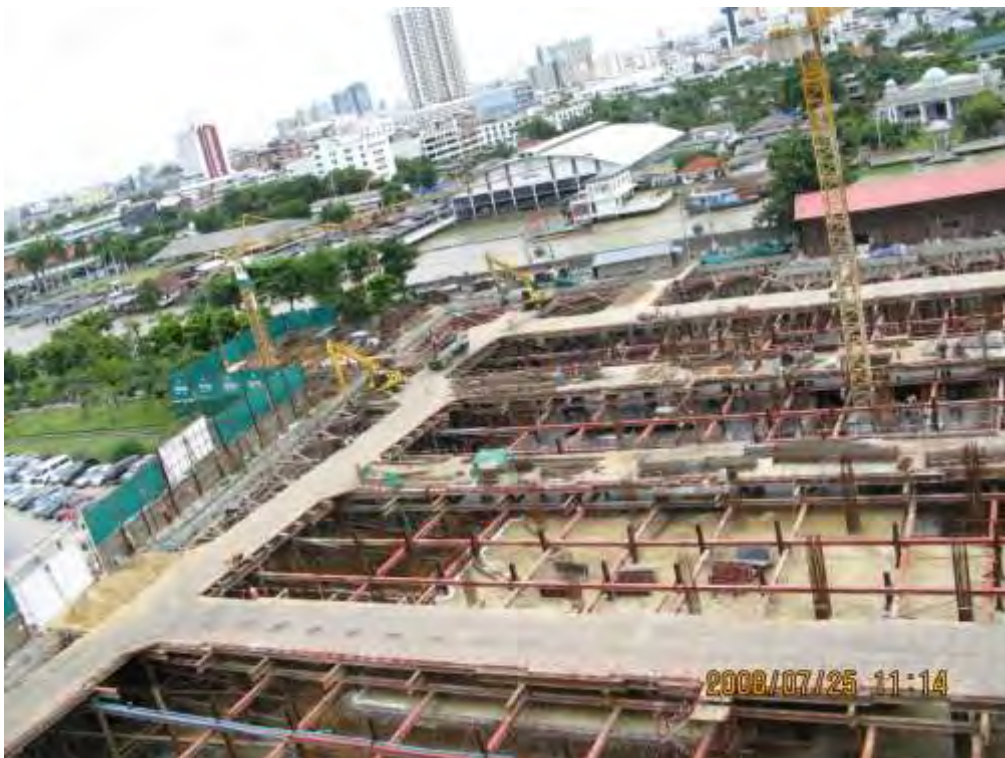
Figure 16 (a). The photographs of the basement construction by means of the contiguous pile wall
