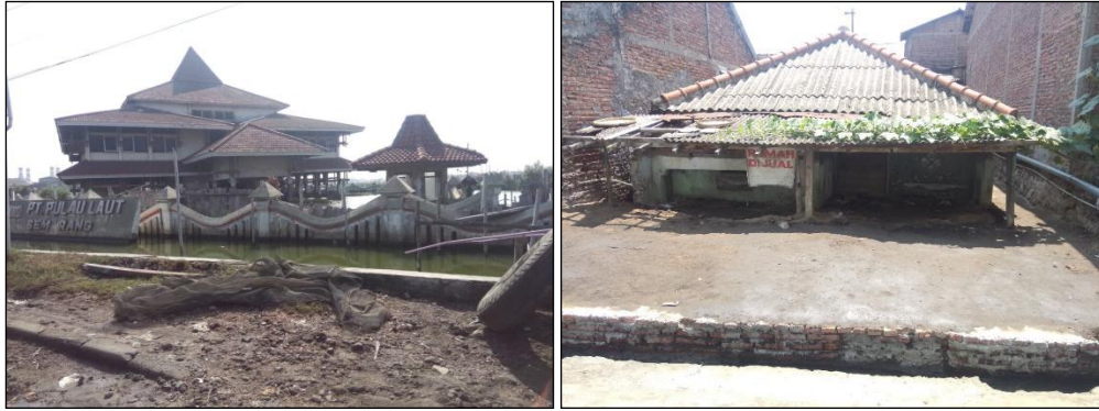
Figure 6. Coastal flooding (in the left) and land subsidence (in the right) in the study area (Source: Field visit, August 2015)
