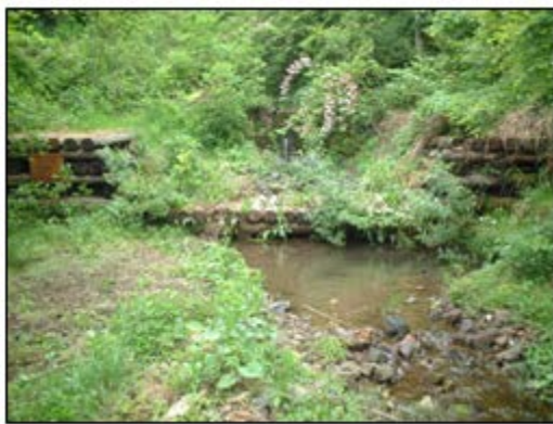
Photo 5. Growth of vegetation on dam
