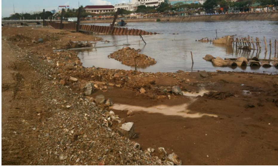
Figure 5. A sliding of the Long Xuyen riverbank under construction of a stabilized structure in an Giang on May 15th, 2012
