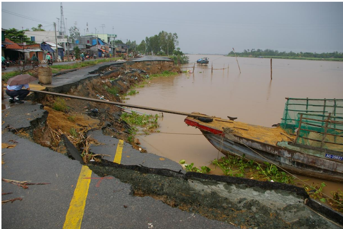
Figure 2. A sliding at km 88 + 937 on the national highway No. 91 along the Hau riverbank in Binh My, An Giang on March 22 nd , 2010
