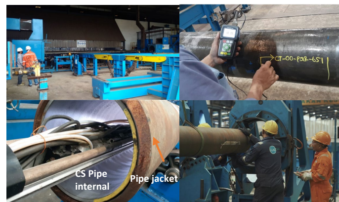
Figure 5 Surface preparation and cleaning by blasting pipe internal (a) UT Thickness check of CS Pipe before welding (b), setting material (c) and start weld overlay cladding (d).
