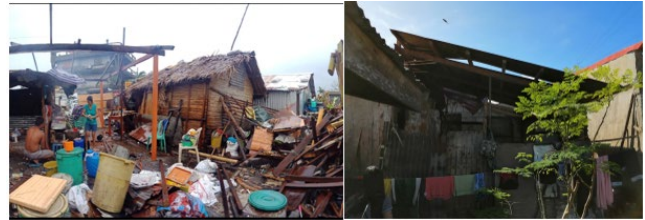
Figure 11 Photos of some of the surveyed buildings that exceeded the maximum damage ratio
