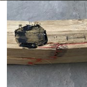
Figure 9. Simple tension & splintering tension failure mode
