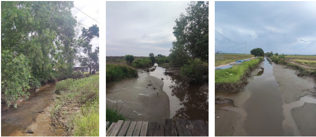
Figure 2 Sedimentation on secondary canals
