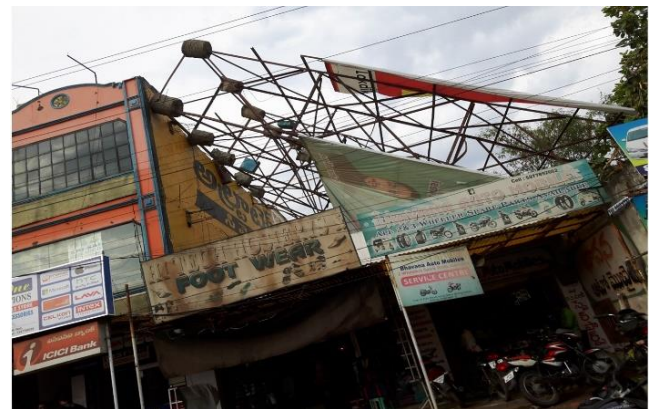
Figure 3 Damage of Billboard and partial damage of building (Raidurgam, Hyderabad, 20 May 2016)
