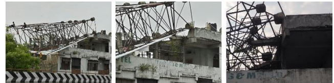
Figure 2 Damage of Billboard and partial damage of building (Langarhouse, Hyderabad, 17 April 2016)
