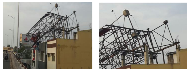
Figure 5 Damage of Billboard and partial damage of building (Tolichowki, Hyderabad, 20 May 2016)
