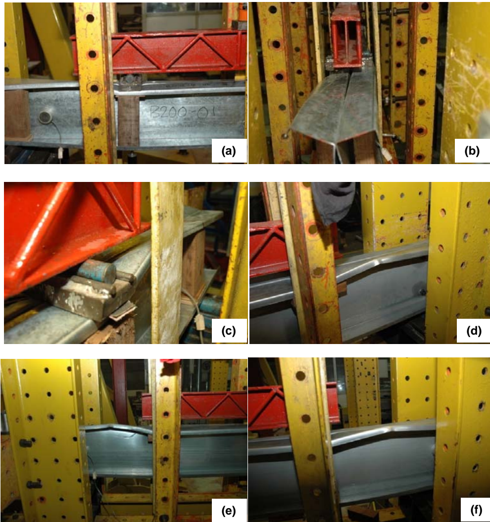
Figure 5 Failure mode (local buckling at top flange) for all tested beams (a) DC200-01 (b) DC200-02 (c) DC200-03 (d) DC250-01 (e) DC250-02 (f) DC250-03
