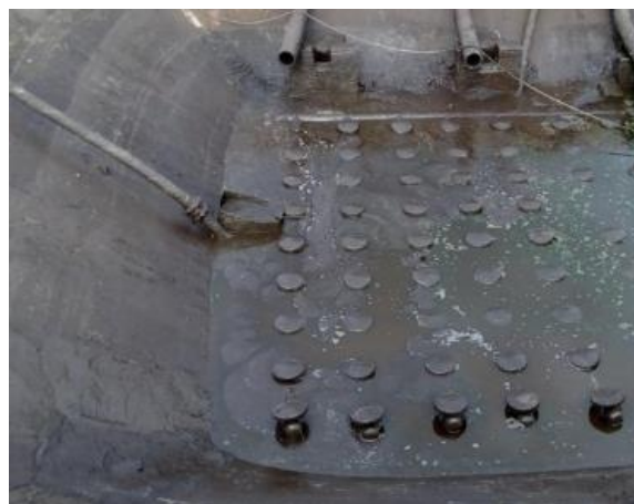
Figure 1 Clogging of diffuser
