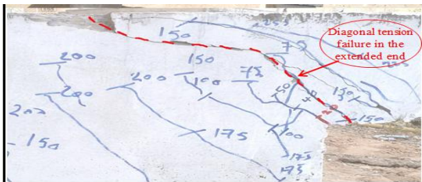
Figure 14 Crack pattern for specimen NCONT-B
