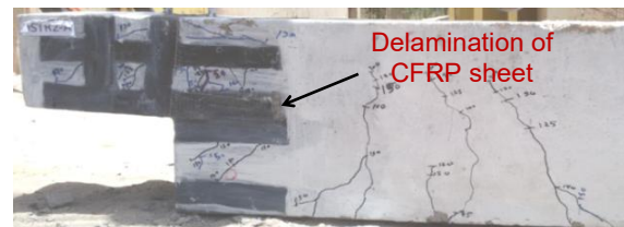
Figure 23 Cracks patterns for strengthening beams NSTR2-A
