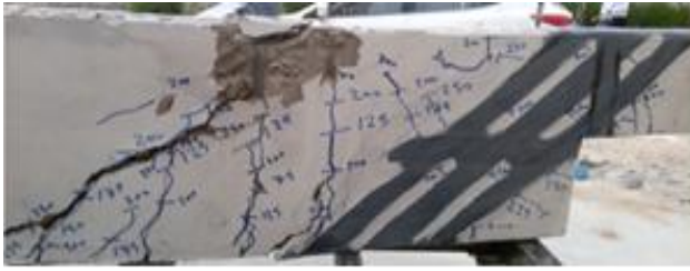
Figure 16 Cracks patterns for strengthening beams HSTR1-A
