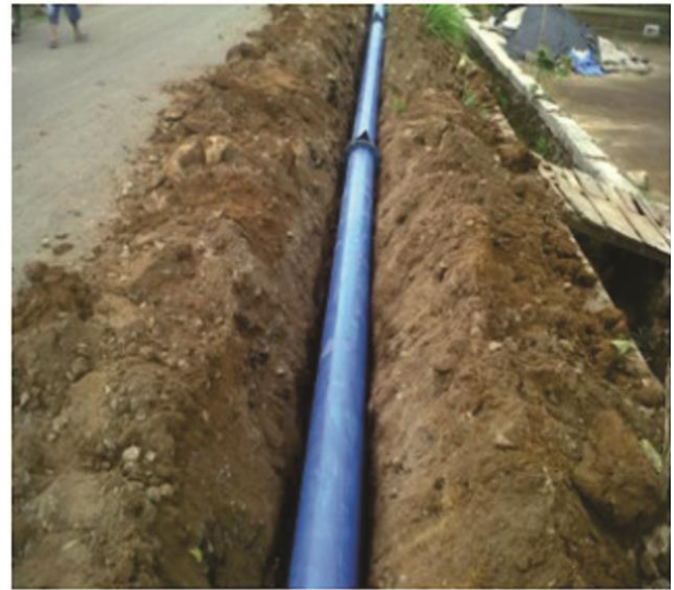
Figure 2 Buried water supply carbon steel pipelines on Sekincau-Way Tenong West Transect Road [2]
