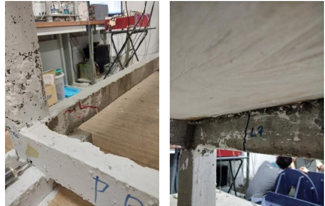
Figure 10 Propagation of cracks in Test 7
