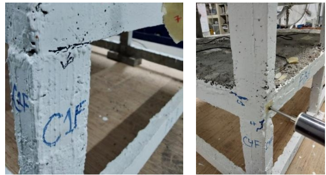
Figure 6 Horizontal and diagonal minor cracks observed at storey 1 in Test 3
