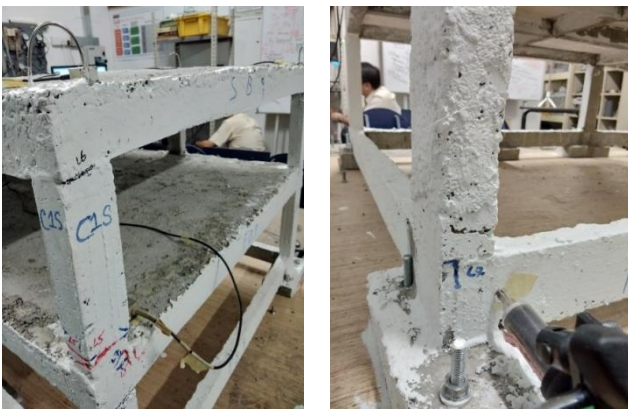
Figure 7 Horizontal and vertical cracks in columns of base and storey 2
