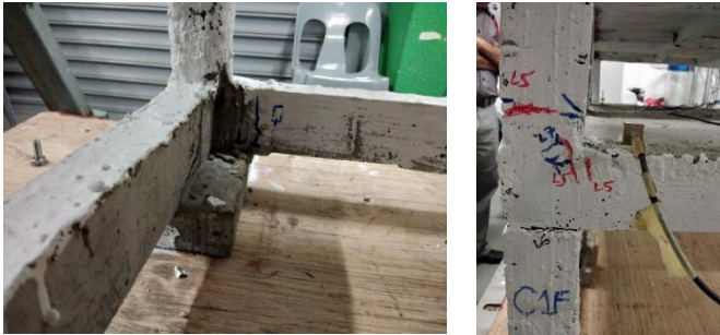
Figure 8 Significant crack patterns at base and storey 1
