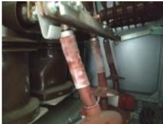
Figure 1 Cubicle Condition Due to Corona Discharge
