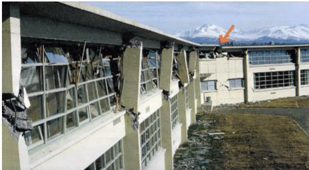
Figure 1 West Anchorage High School in Alaska sustained damage to its roof diaphragm at the re-entrant corner during the 1964 earthquake [11]
