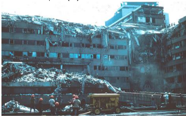
Figure 2 The upper floors and re-entrant corner of Mexico City's Ministry of Telecommunications Building were damaged during the 1985 earthquake [12]
