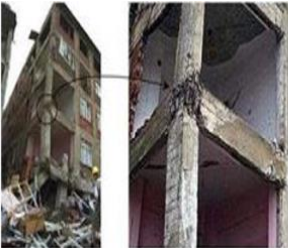
Figure 1a Joint Failure
