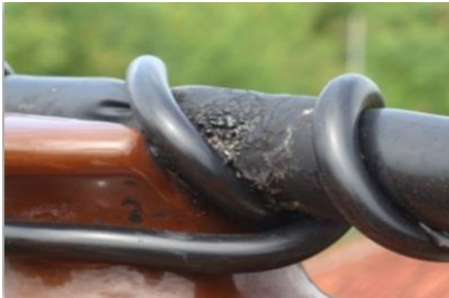
Figure 1 Sheath degradation of AAAC-S
