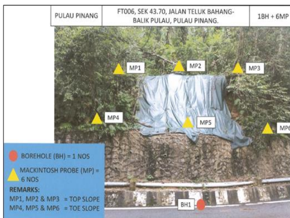
b) Landslide FT006 S43.70
