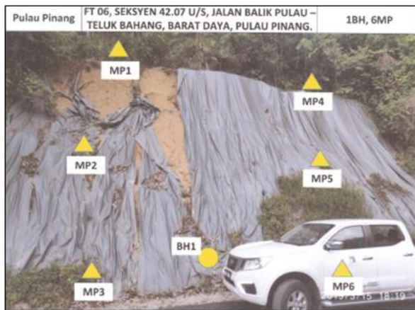
a) Landslide FT006 S42.70
