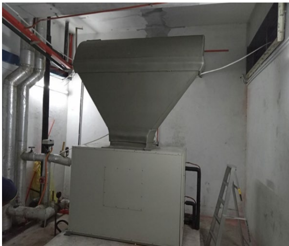
(b) Multi-circuit Air conditioning unit
