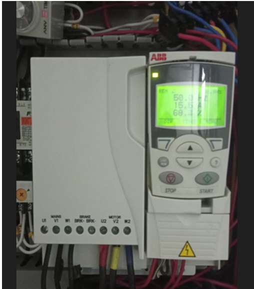
(c) Variable frequency drive for compressor 1
