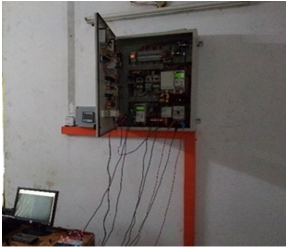
(a) Power and Control unit
