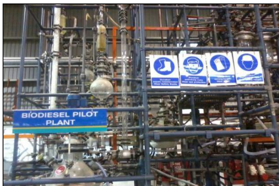
Figure 3 Biodiesel pilot plant
