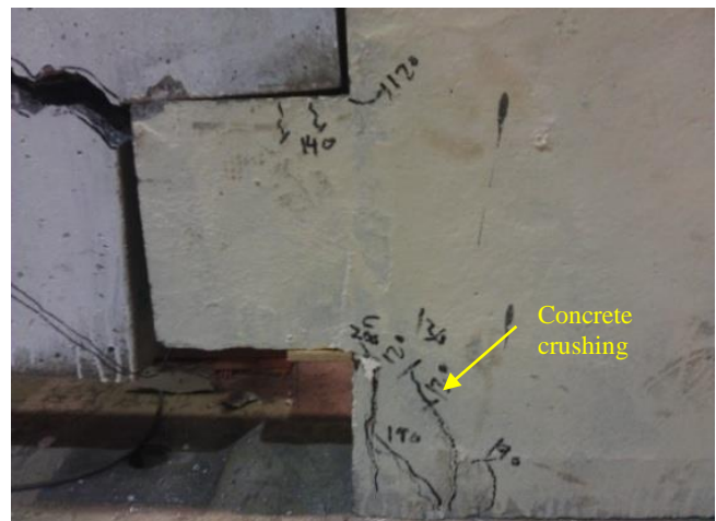
Figure 8 Crushing of corbel support
