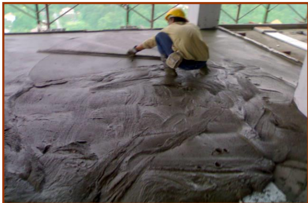
Figure 1 Lightweight foamed concrete been poured in sections to prevent loss in density and reduce shrinkage problems in slabs for UEM building project in Kuala Lumpur, Malaysia
