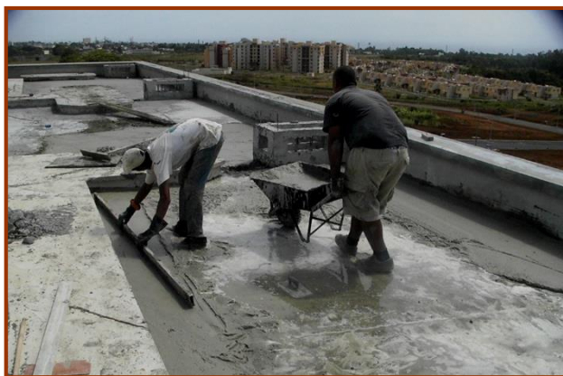
Figure 2 Lightweight foamed concrete insulation screed was utilized to offer thermal protection for a multi storey building in Mauritius
