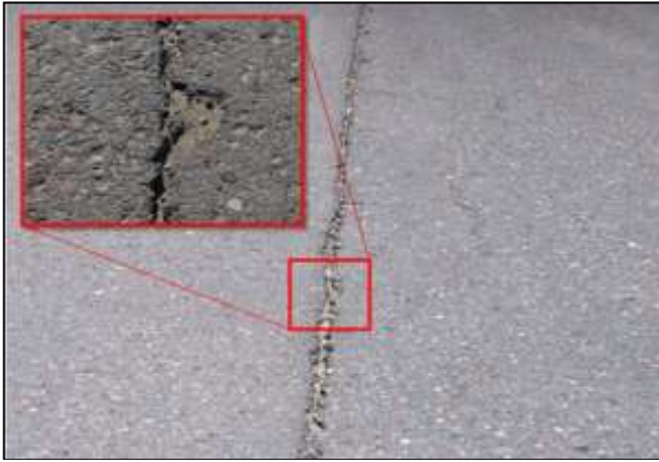
Figure 2 Longitudinal joint crack opening filled by undesired materials
