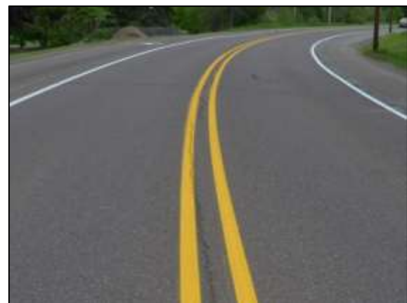
Figure 1 Longitudinal joint cracks
