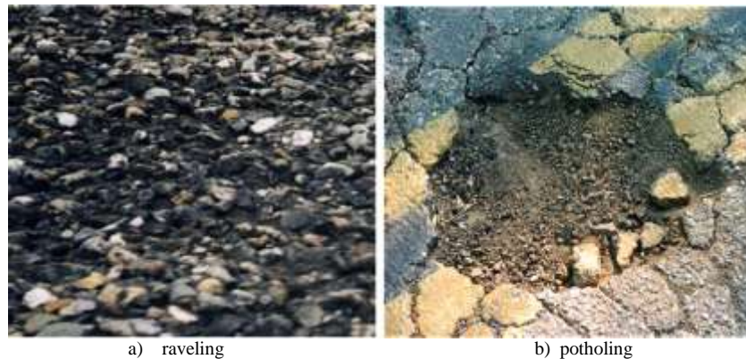
Figure 2 Moisture induced damage in asphalt mixture [36]
