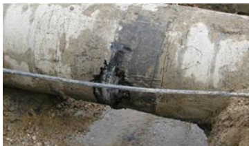
Figure 1 Example of deformation damage (wrinkle probably caused by landslide) [12]
