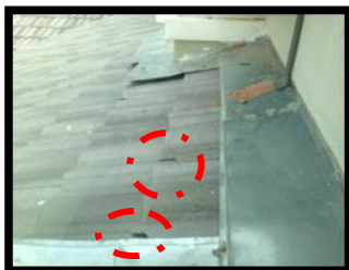
Figure 9 Broken roof tiles
