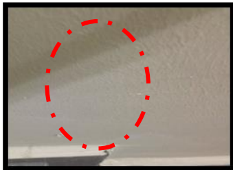
Figure 5 Wall surface rough
