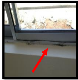
Figure 17 Window frame filts/damaged
