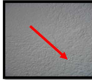
Figure 10 Rough wall Surface and cracks
