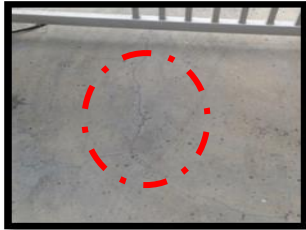
Figure 3 Cracks in floor
