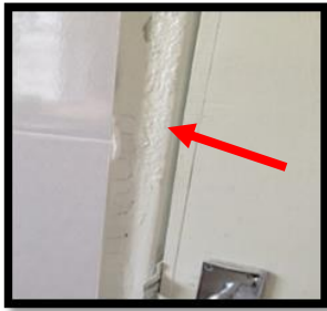
Figure 16 Cracks / flaking painting in door frame
