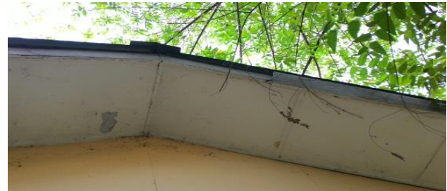
Figure 4 Peeling paint on the soffit board
