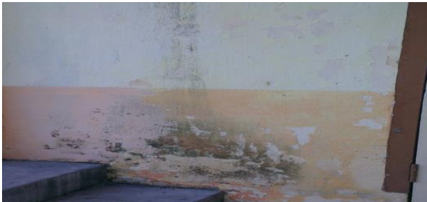
Figure 5 Mould growth on the wall
