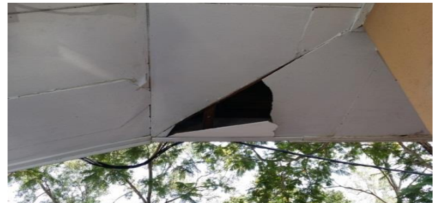
Figure 3 Damaged of the soffit board
