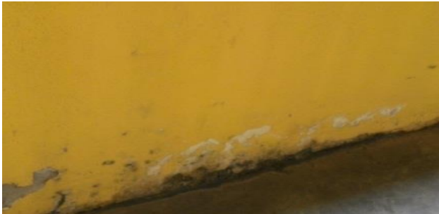
Figure 6 Minor peeling paint on the wall
