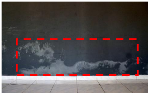
(a) Rising damp clearly seen at the base of the wall
