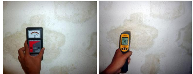
Figure 1 Moisture meter (left) and Infrared Thermometer (right) intact with dampness area
