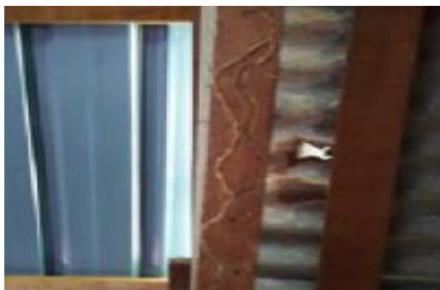
Figure 9 Termites nest on the column area
