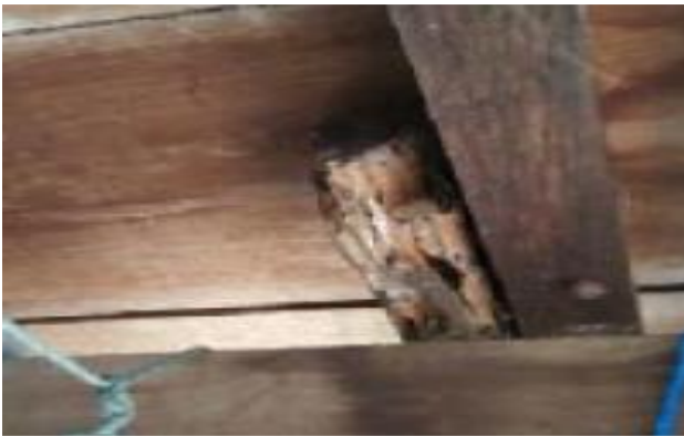
Figure 2 Decay of timber underneath floor slab
