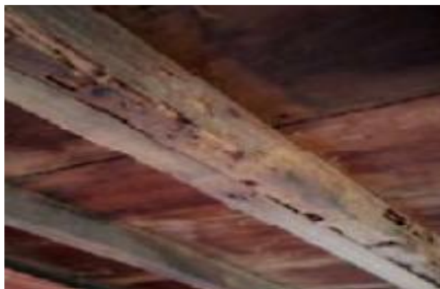
Figure 8 Deterioration of timber beam
