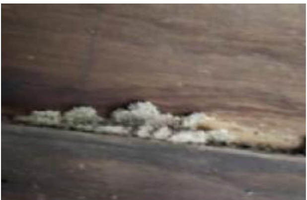
Figure 3 Termites attack on beams at 1 st floor
