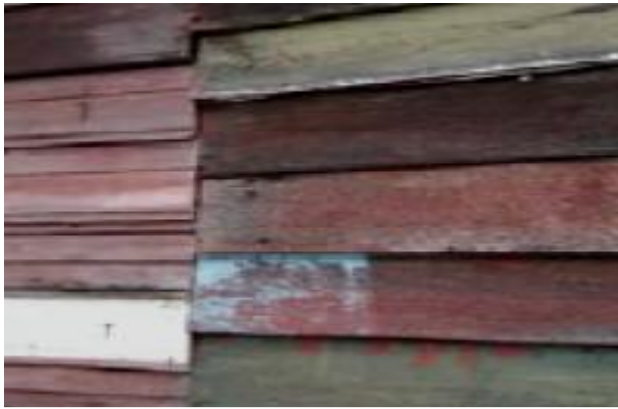
Figure 10 Discoloration of timber wall
