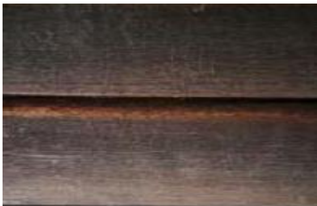
Figure 7 Discolouration of timber
