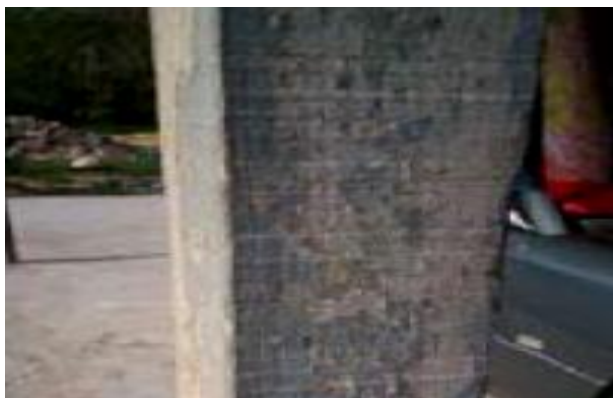
Figure 6 Scaling of painting at column area
