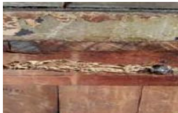
Figure 5 Deterioration of timber
