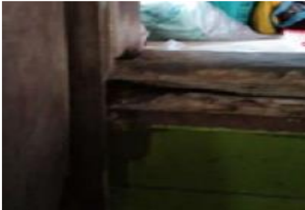
Figure 1 Deterioration of timber window frame
