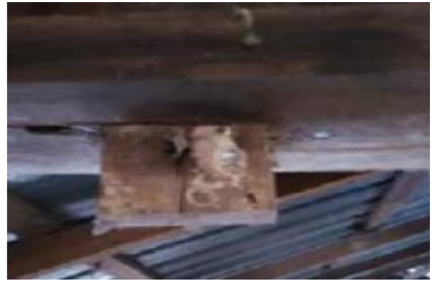
Figure 4 Insect attack from beetles on timber roof section
