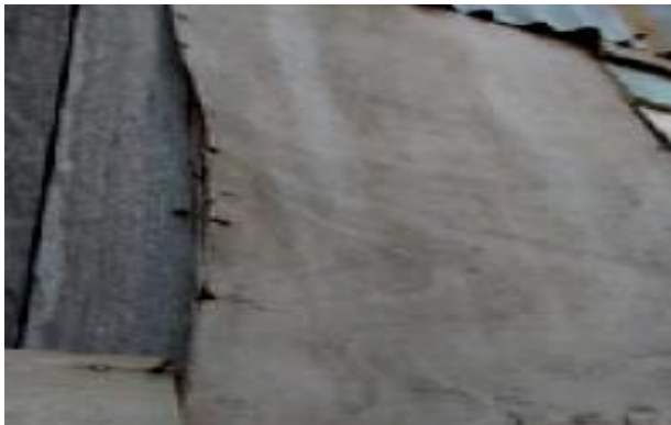
Figure 11 Warping of timber partition
