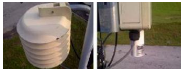
Figure 2 Outside temperature sensor and humidity sensor
