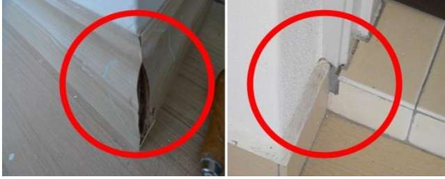
Figure 5 Defects at the wall skirting
