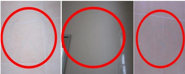
Figure 6 Hollowness in the wall tiles.
