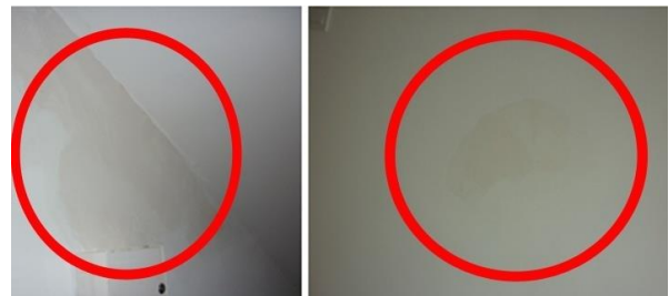
Figure 8 Unevenly applied wall paint.
