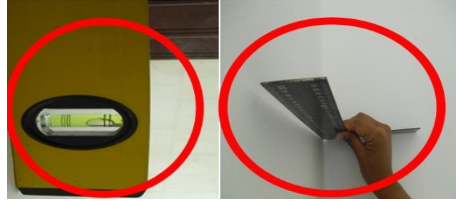
Figure 7 Walls angled incorrectly
