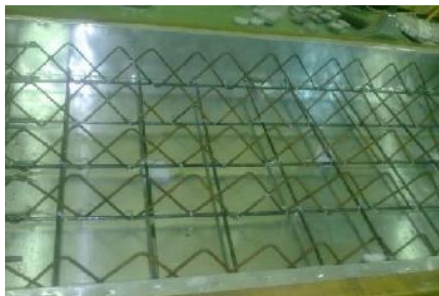
Figure 1 Double Shear truss connectors tied to steel bar reinforcement in PLFP panel
