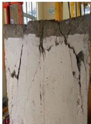
Figure 6 Crack and crush on the diagonal angle approximately 45° at the top of panel PC-3
