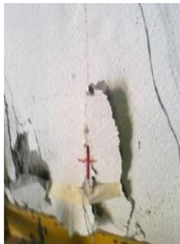
Figure 5 Crack and crush at bottom part of panel PA-1
