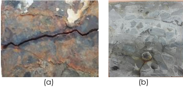
Figure 4 Cracking pattern at longitudinal direction (a) and the lateral direction (b)
