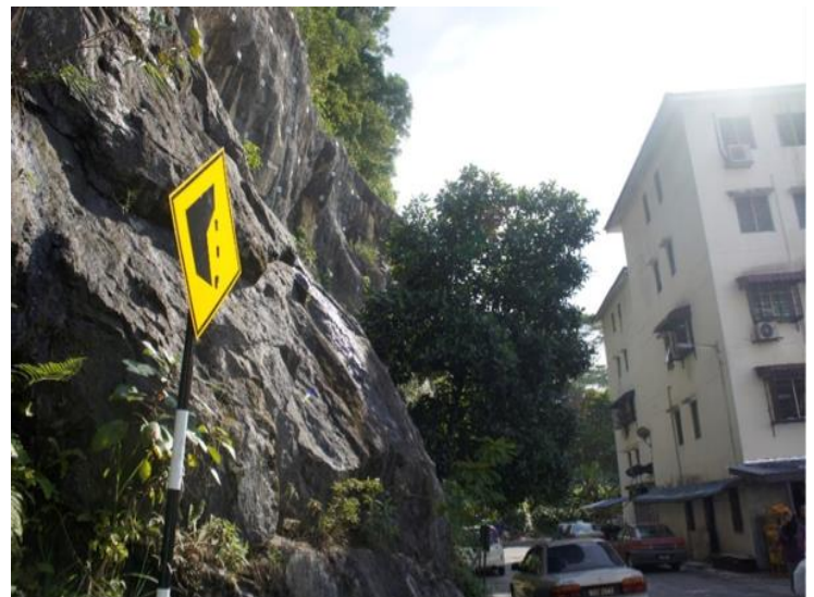
Figure 3 Pangsapuri Intan was built close to the unstable rock slope. (note: the rockfall signboard)
