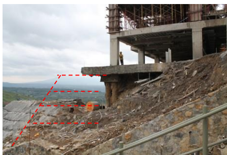
Figure 2 Landslide case in the Sport Training Center project at Hambalang Sentul, West Java [3]
