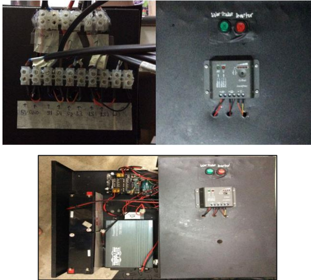
Figure 19 Controller Box Connection, Batteries, and Inverter
