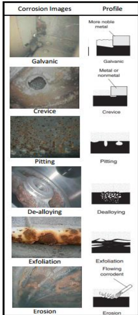
Figure 2 Corrosion image with profile.
