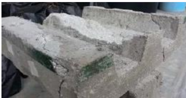
Figure 19 The condition of the control sub-panel after dismantling
