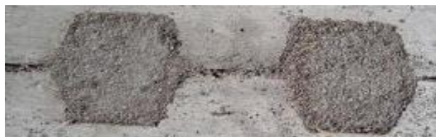
Figure 15 The condition of the infill material of FRLFC
