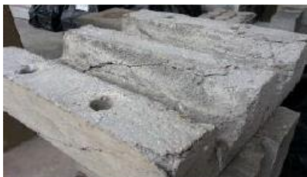
Figure 20 The condition of the FRLFC sub-panel after dismantling
