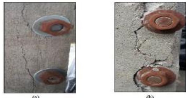
Figure 13 (a) Small cracks on the surface of FRLFC (b) Wide cracks on the control specimen
