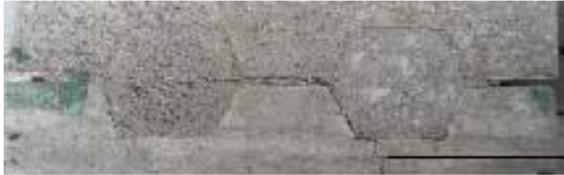
Figure 14 The condition of the infill material of the control LFC wall panel
