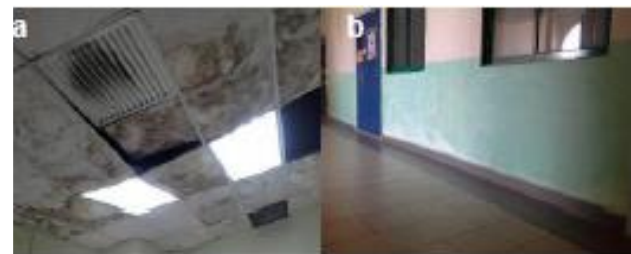
Figure 10 Deterioration due to Condensation and Moisture problem: (a) Microbial Growth on Ceiling and (b) Failure of Paints on Walls
