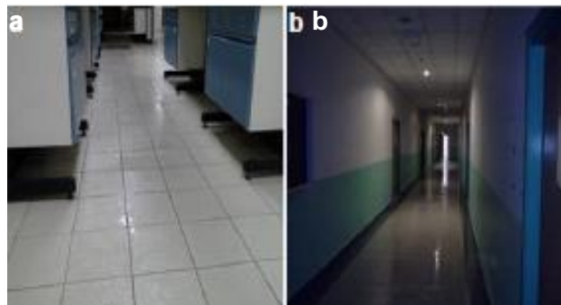
Figure 6 Condensation on floor in non-air-conditioned spaces sitting over plenum return air-conditioned space
