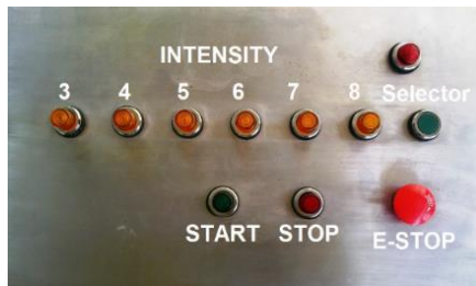
Figure 9 Control panel with start, stop, e-stop and intensity buttons from III to VIII
