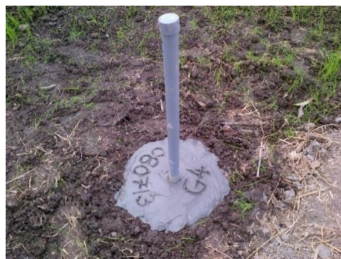
Figure 2 Monitoring well for groundwater sampling
