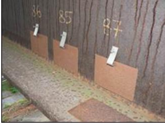
Figure 6 Darker patina layer about 50 mm above the bottom flange on external web of northern main girder
