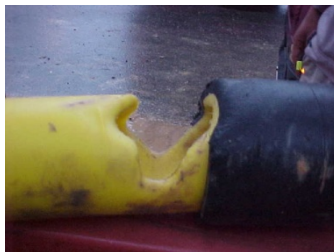
Figure 5 Damaged MDPE gas pipe showing serious shear remnants of sand blasting impact
