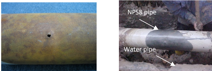
a. Oxidized NPS8 carbon steel pipe indicating leak section b. NPS8 carbon steel pipe at incident site
