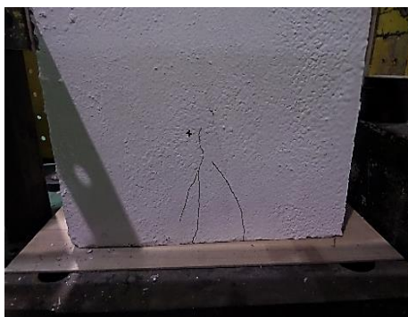
(a) Cracks on the slab surface
