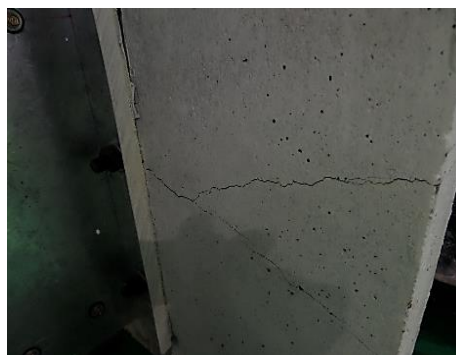
(b) Cracks underneath the slab
