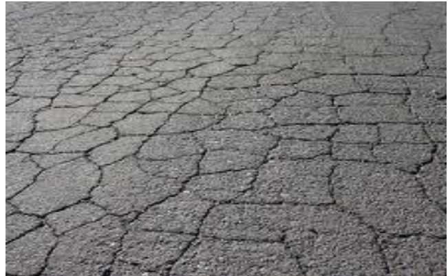
Figure 6 Fatigue cracking encountered on pavement
