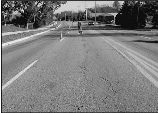
Figure 1 First Stage of Top-down Cracking
