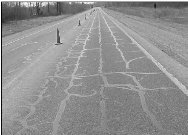
Figure 3 Third Stage of Top-down Cracking
