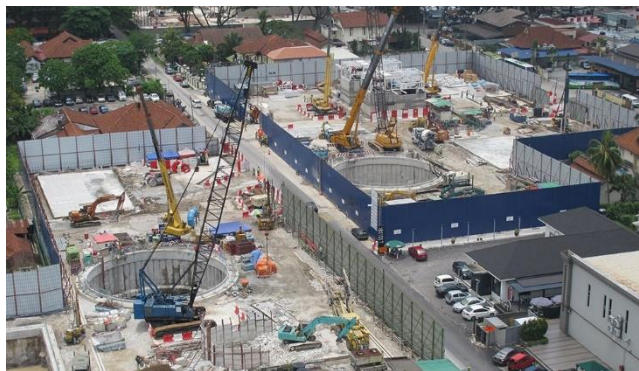
Figure 10 Overall view of the two completed TBM launching shafts (picture sourced from internet).
