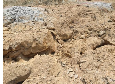
Figure 10 The rock split in lines 2 and 3 and not moved far
