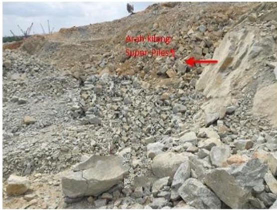
Figure 8 Inspection carried out on site. Red arrow indicates the direction of joint dominance (to the west)
