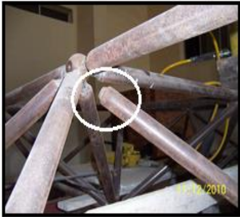
Figure 28: Collapse in connections (20&23) from the third test of truss#1
